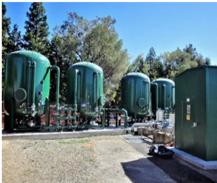
Granulated Activated Carbon (GAC)
