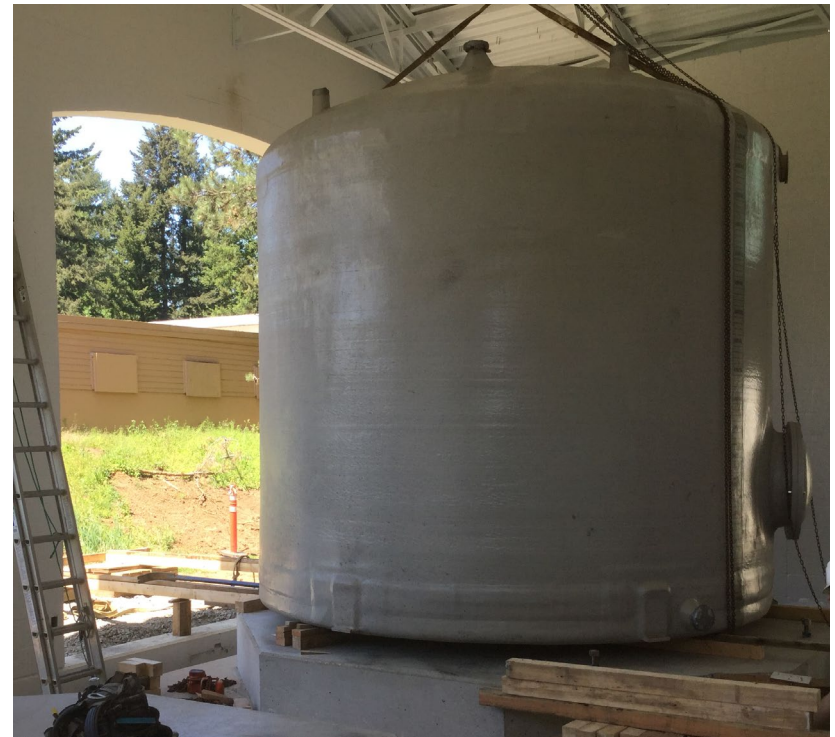
Water Station 1 tank installation example
