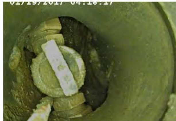
Non-Lead Service Line
