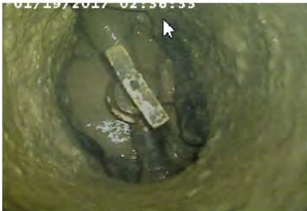
Lead Service Line
