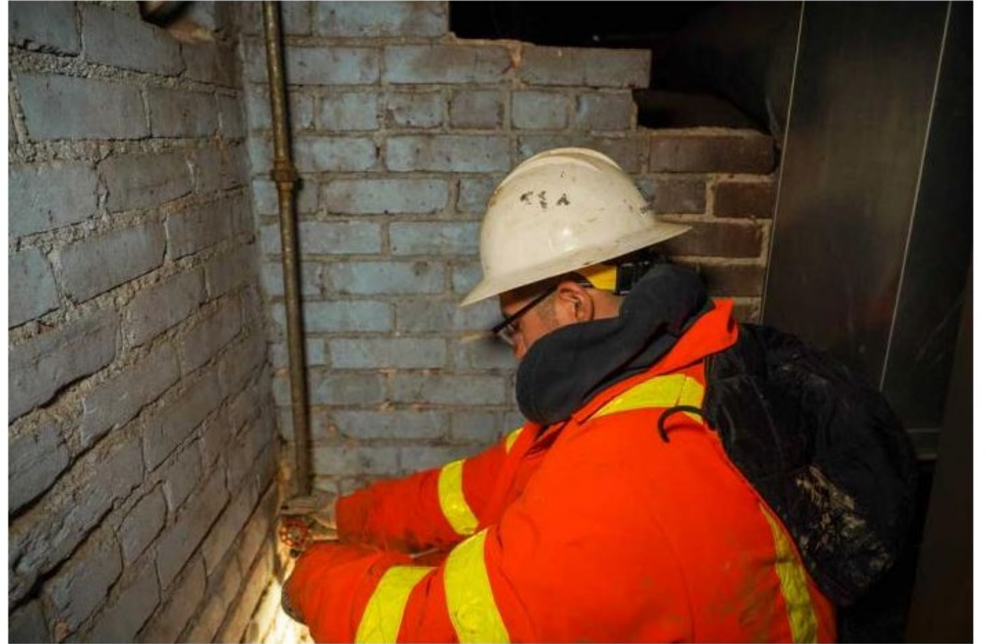
Denver Water field crews or its contractors may inspect the pipe at the main water shut-off valve inside the property to help determine the type of material. Visual inspection will be arranged with the property owner in advance. Photo credit: Denver Water.
