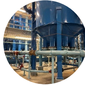
Activated Carbon Treatment
