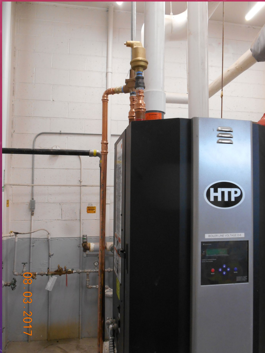
Hot Water Loop & Boiler
