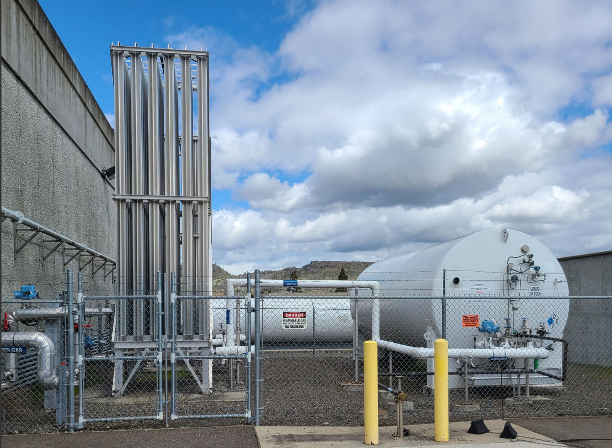
LOX Tank and Vaporizers
