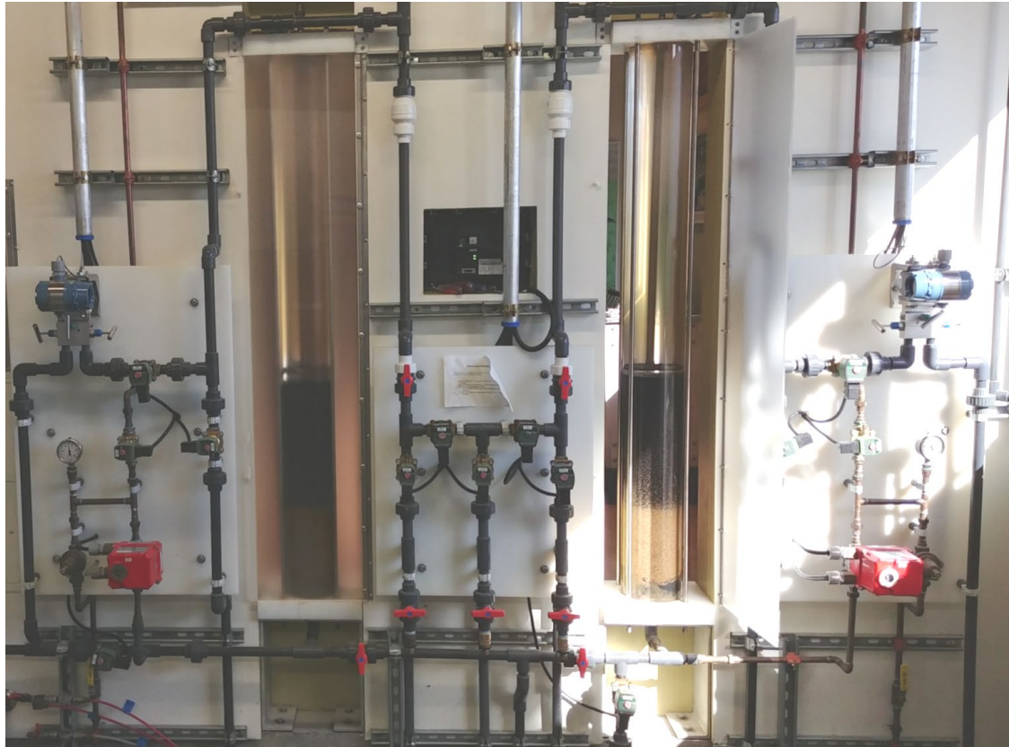
Control and Chlorinated Pilot Filters
