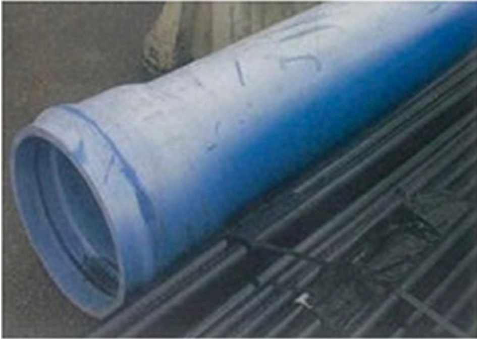
Figure 1: Surface discoloration of PVC pressure
