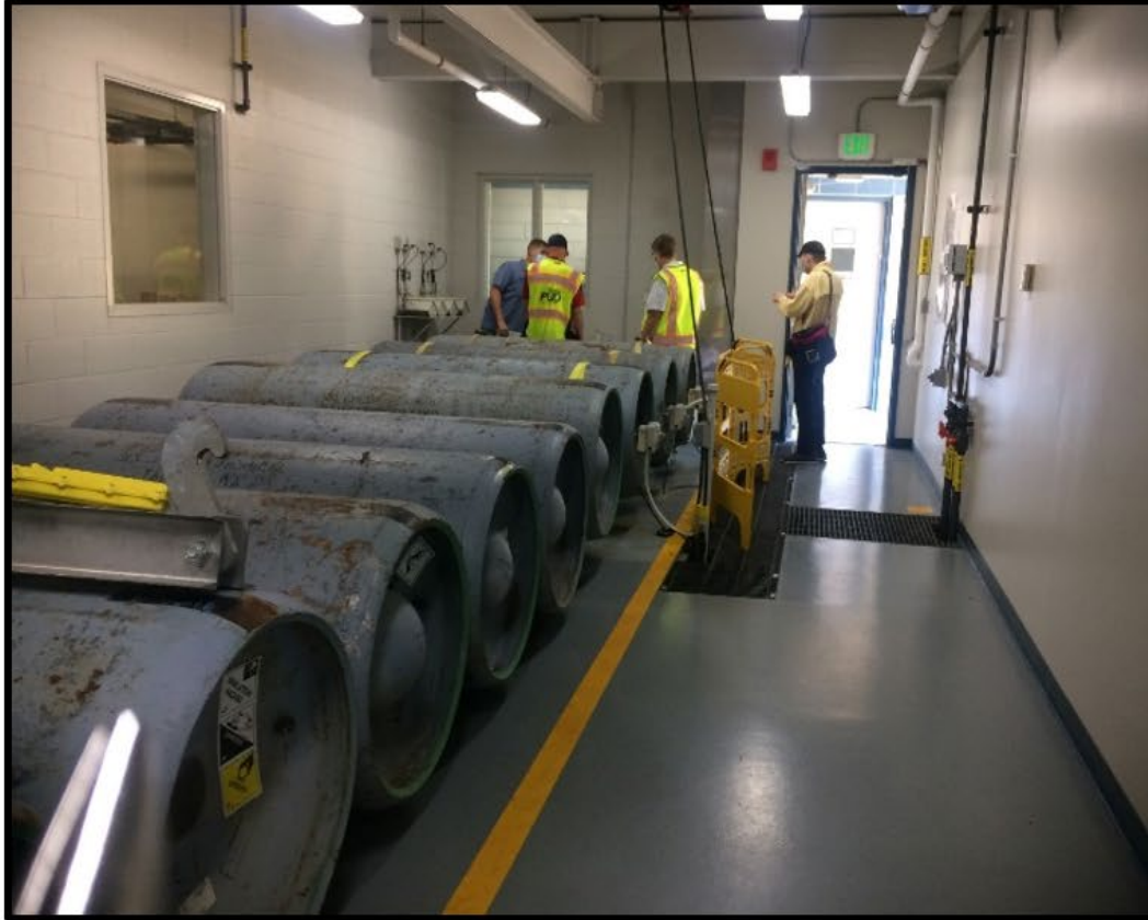
Figure 1-3. Chlorine Cylinder Storage Room
