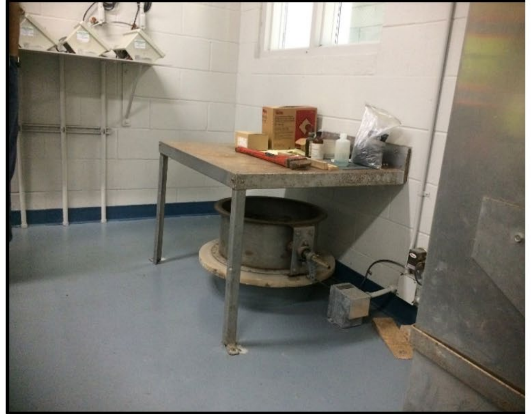
Figure 1-4. Existing Exhaust Duct and Damper
