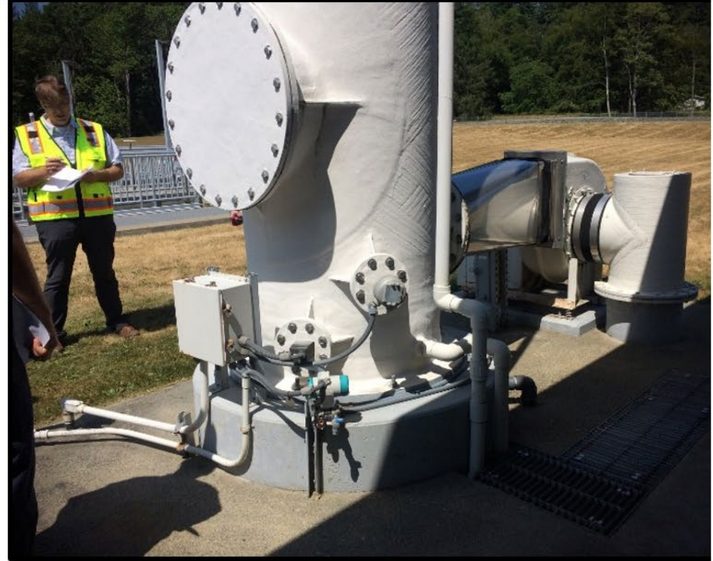
Figure 1-2. Existing Chlorine Scrubber and Exhaust Fan
