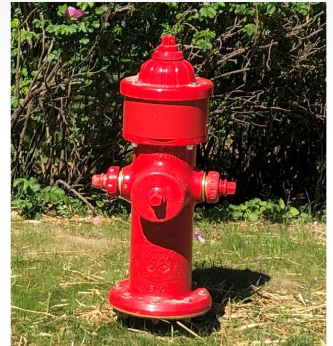
iHYDRANT® | INSTALLATION, VERMONT
