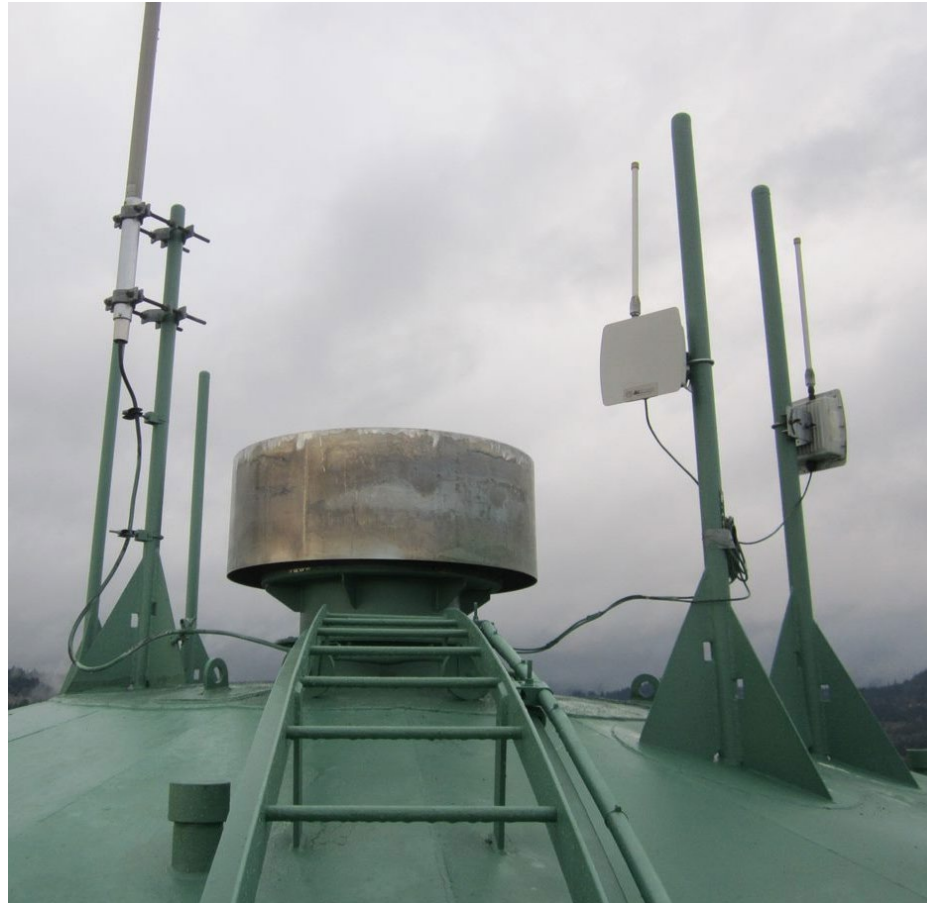
Added Cell Equipment Supports
