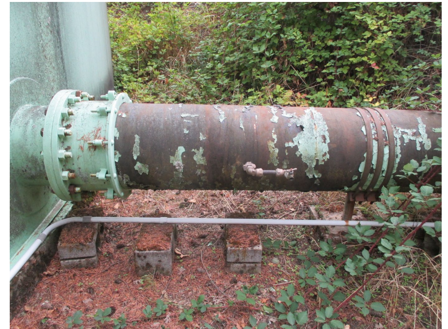
Typical Unrestrained Flexible Coupling on Piping at Reservoir Footing
