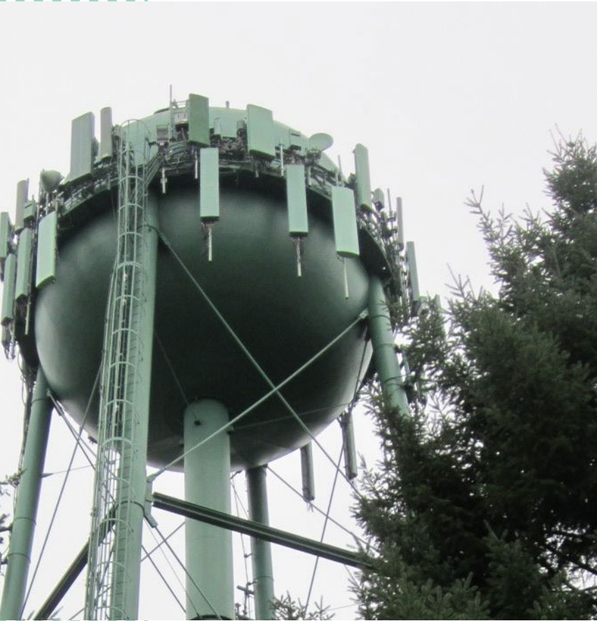
Extensive Cell Equipment Attached to Catwalk and Railing
