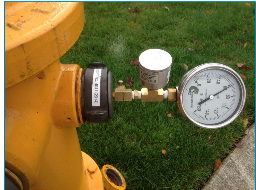
Hydrant pressure transducer
