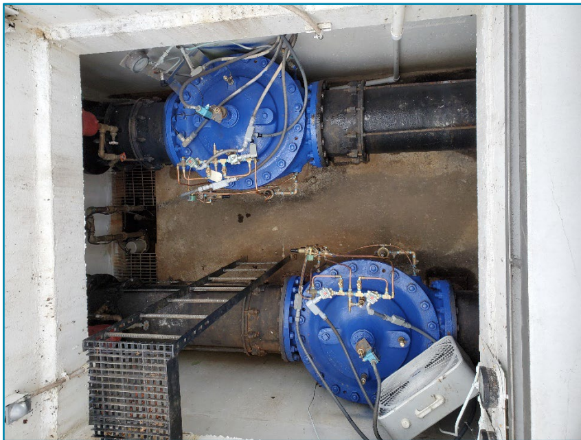
Master meter vault
