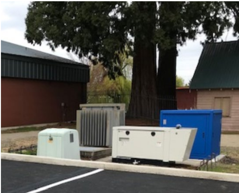
Pump House (Pump Control)
