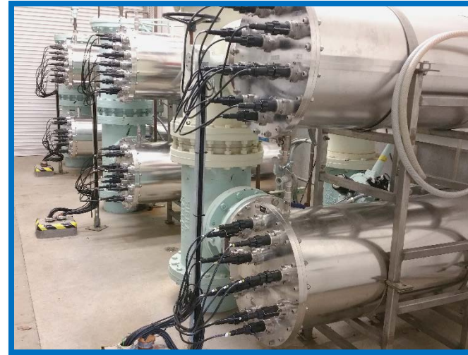
UV Reactors at Canby WTP
