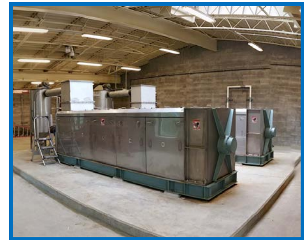
Screw presses at the LO-T WTP
